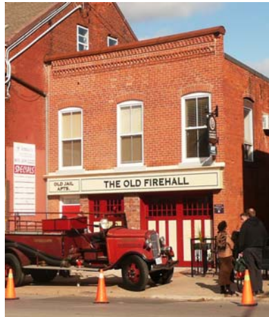
Examples of heritage restorations utilizing photo documentation and heritage resources to match the original façade (above old Firehall in Downtown Grimsby; below Quebec Bank in Downtown Thorold).
