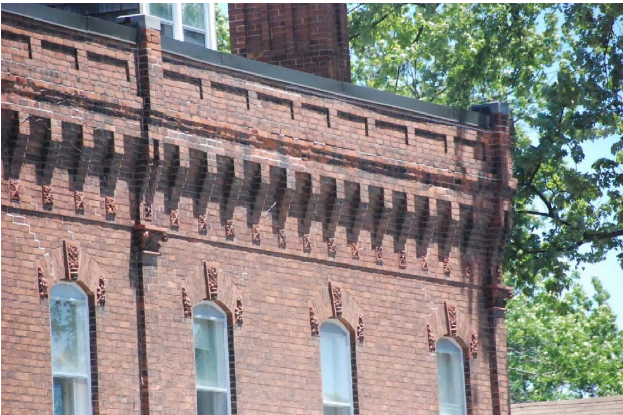
Rooflines with preserved architectural detailing in its original provides a visual attractive “cap” to the top of traditional buildings.
