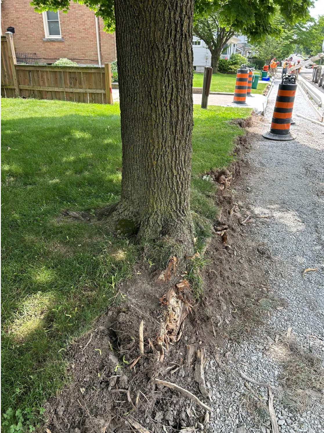
Figure 2 – Tree #2 and damaged roots. Date: June 5 2025.
