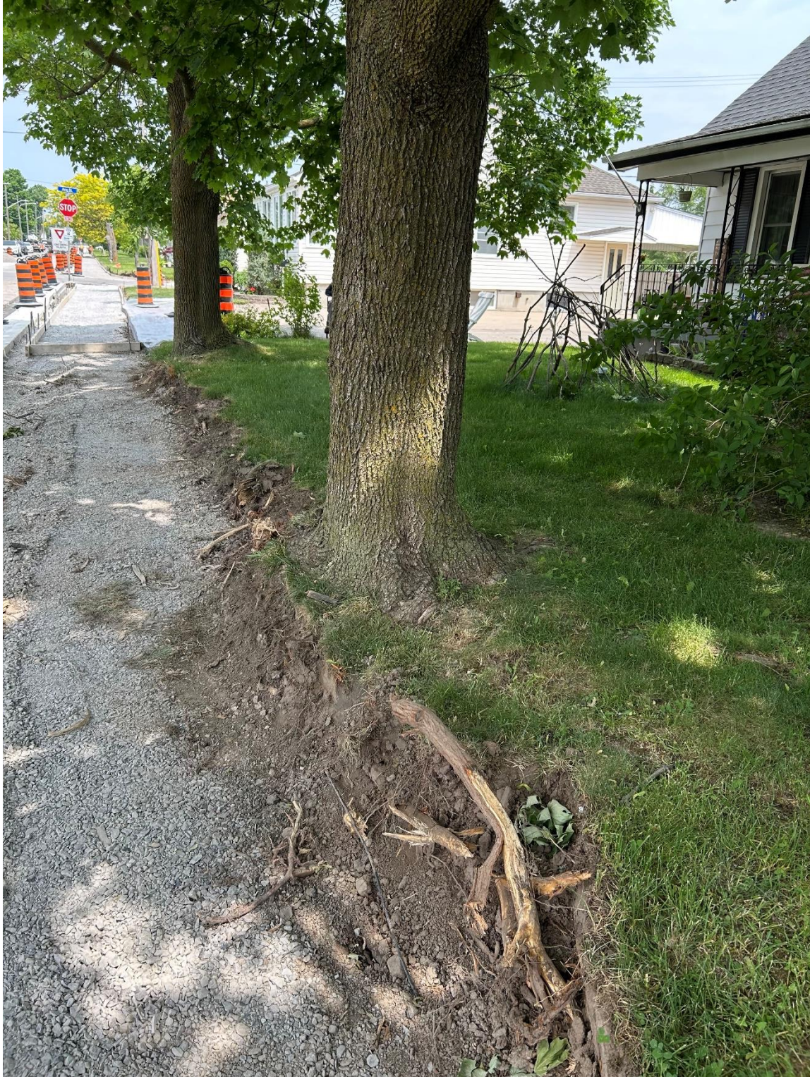
Figure 4 – Tree #1 (left) and Tree #2 (right) with root damage during construction. Date: June 5 2025.
